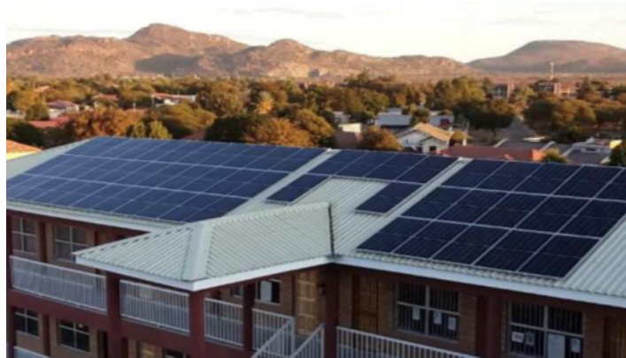
Figure 29: PV installation at Regent Hill International School in Gaborone
