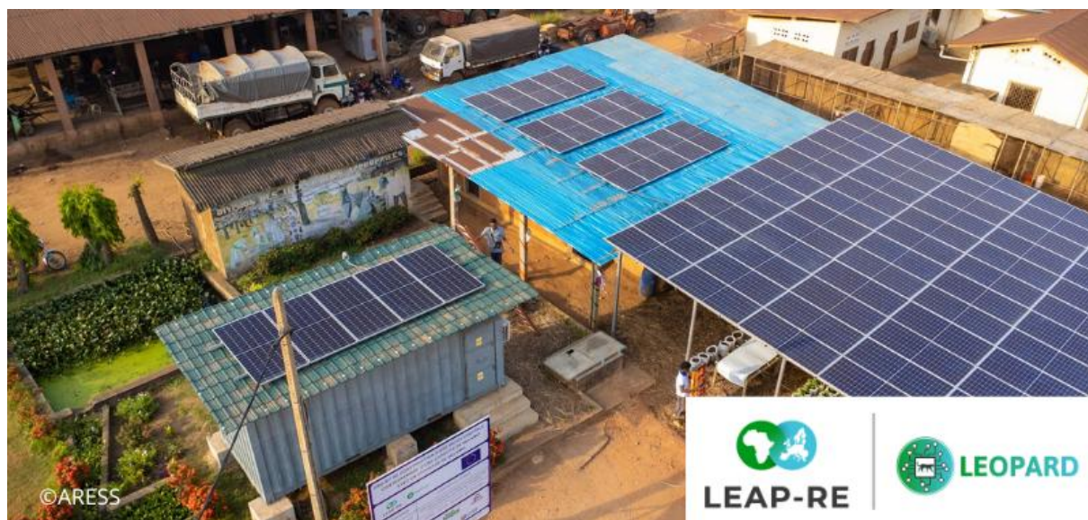
Figure 1: The first LEOPARD demonstrator was installed on the Centre Songhai campus in Benin in 2022.
